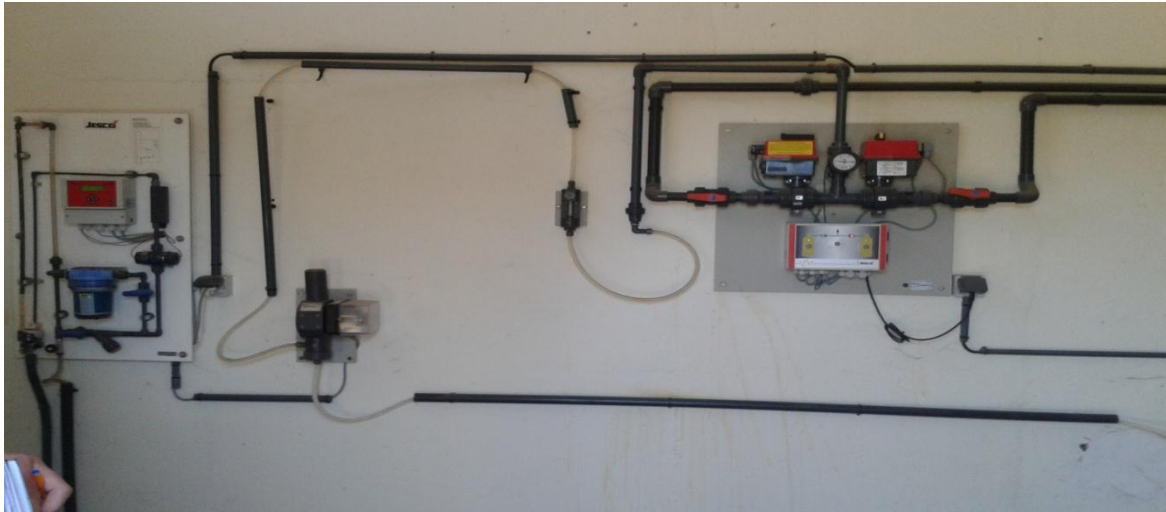
Photo 9 : Station de chloration de km6 Tanks de chlore
