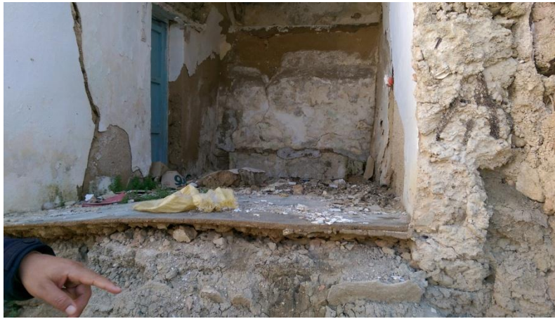
Figure 55 . construction sans fondations
