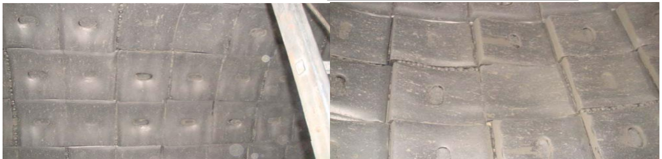
Figure 33-14 : usures blindages releveurs C1
