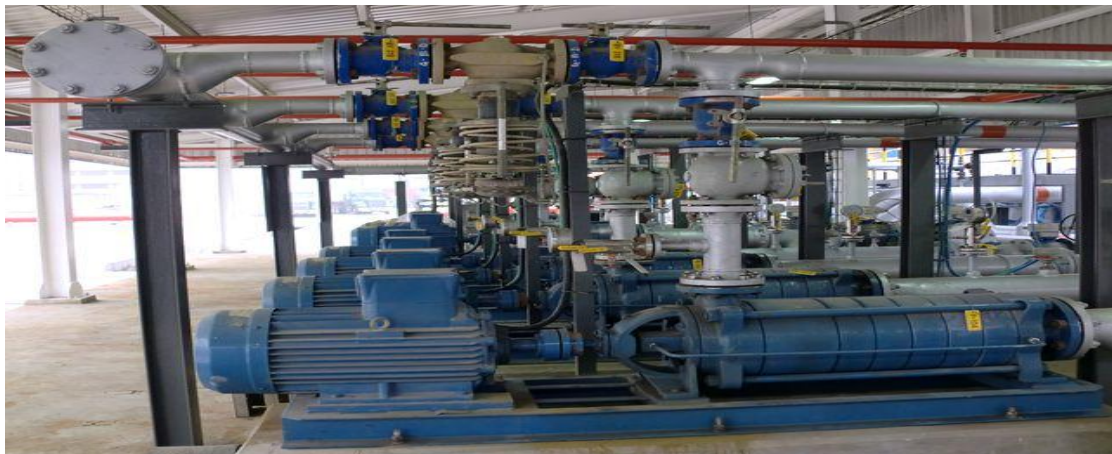
Figure 12 :les Pompes de GPL
