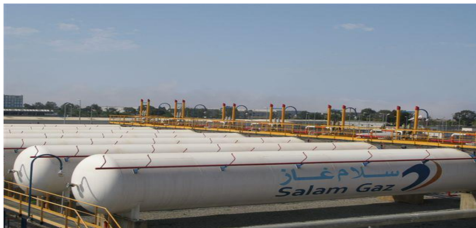
Figure 7 :Stockage de GPL
