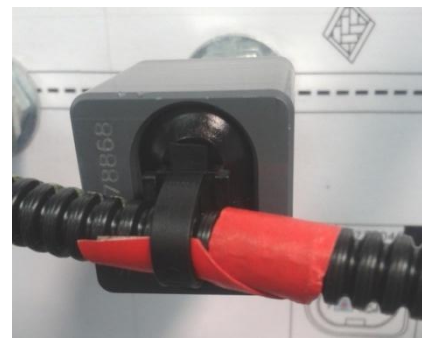
Figure 26: Bride mal serrée
