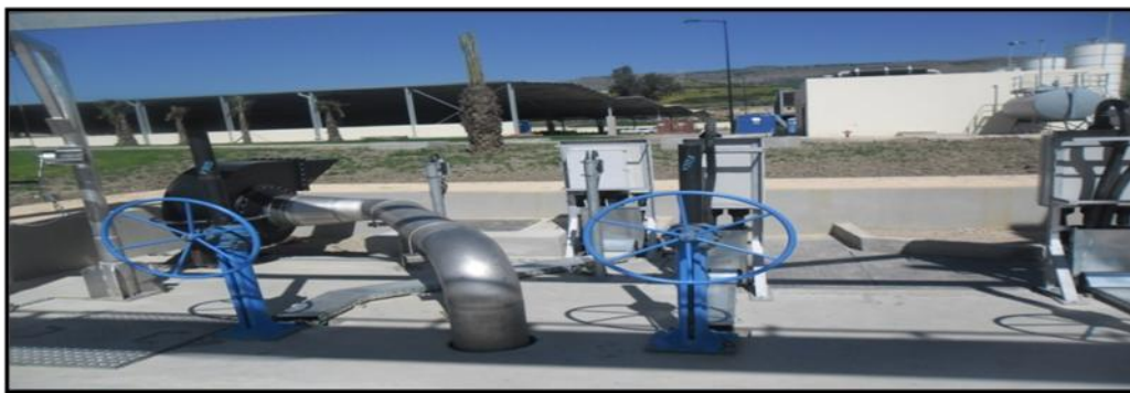
Figure 2: Station de relevage STEP Fès
