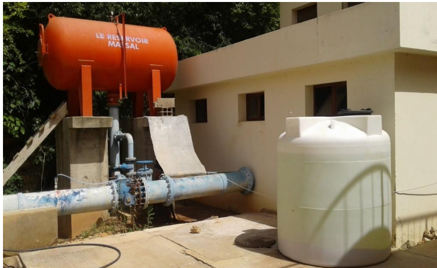
Figure 3 : Station de chloration
