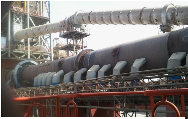
Fig.15: four rotatif a HOLCIM RAS EL MAA
