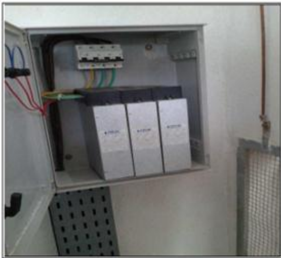
Figure 9: Condensateurs de compensation
