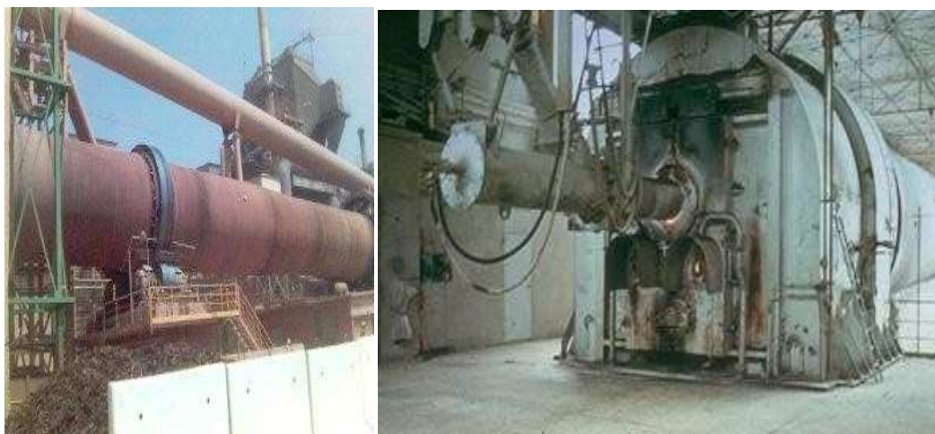
Figure 11-Four rotatif Lafarge- Usine Meknes
