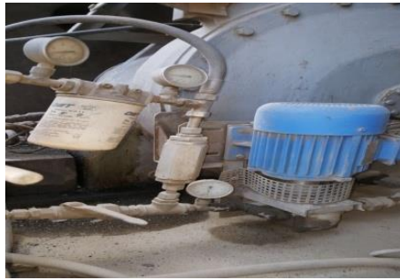
Figure 24: La pompe hydraulique
