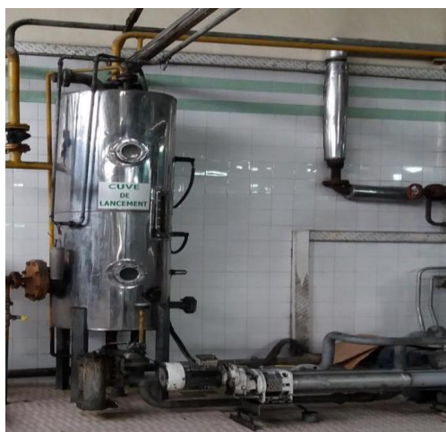
Figure 2: cuve de lancement
