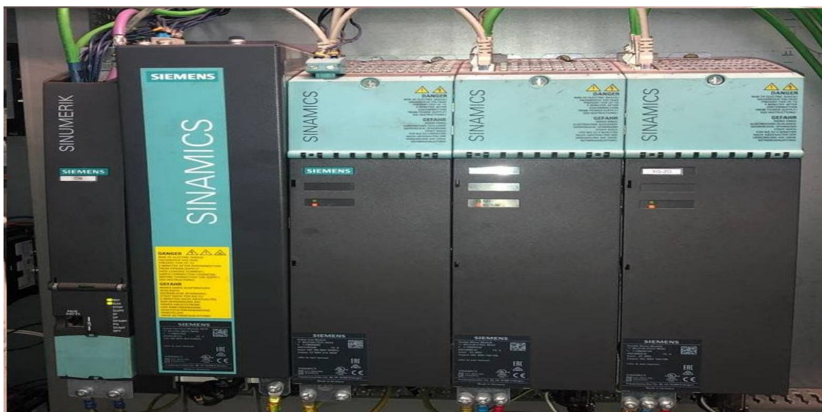
Figure 13: automate de commande.
