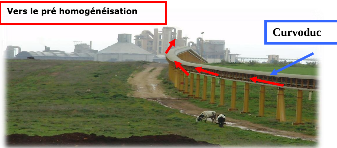
Figure 4: Curvoduc de LafargeHolcim Meknès
