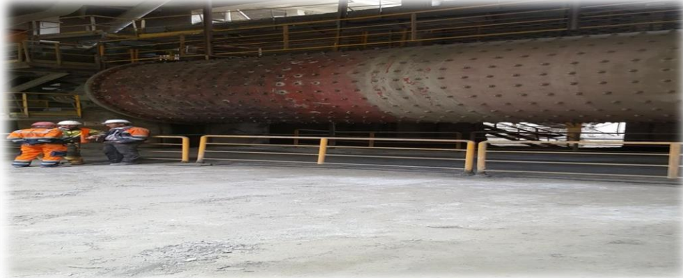
Figure 21: Broyeur ciment (BK)
