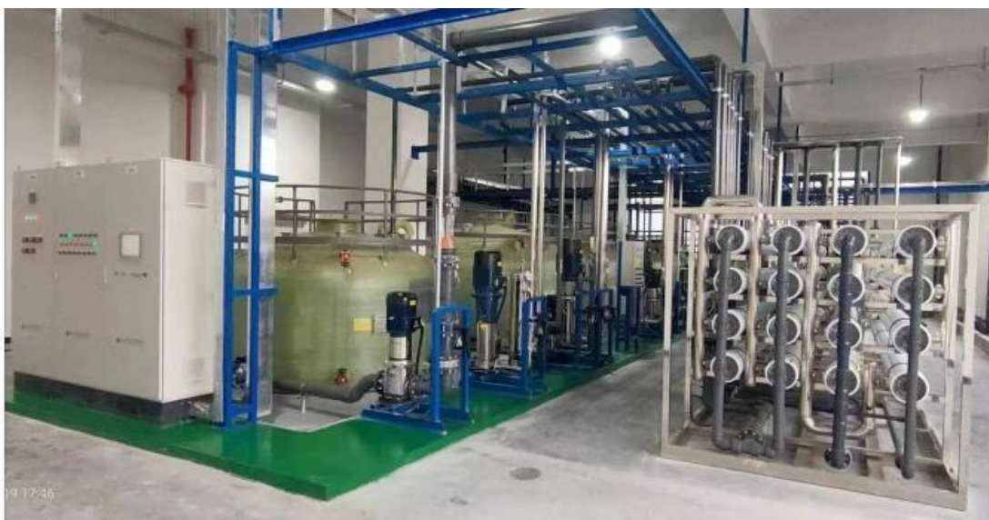
Figure 3 : Station de pompage
