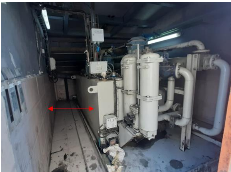
Figure 3.9: Centrale de lubrification de CIMAT
