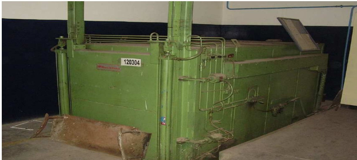
Figure 8: four de stabilisation
