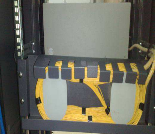
Photo 6: Connections des breakers de IA
