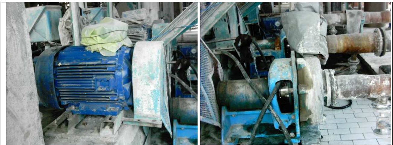
Figure 4-4 : illustration de la pompe acide fort P03
